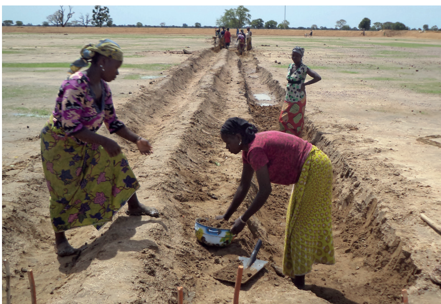
Women from the project helping to build the quaternary canal for their lots.
