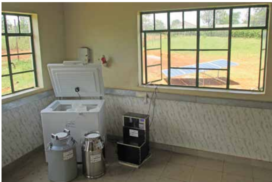
The system consists of PV panels, a commercially available DC freezer equipped with a smart control unit and two insulated milk cans with a 30-litre capacity each.
