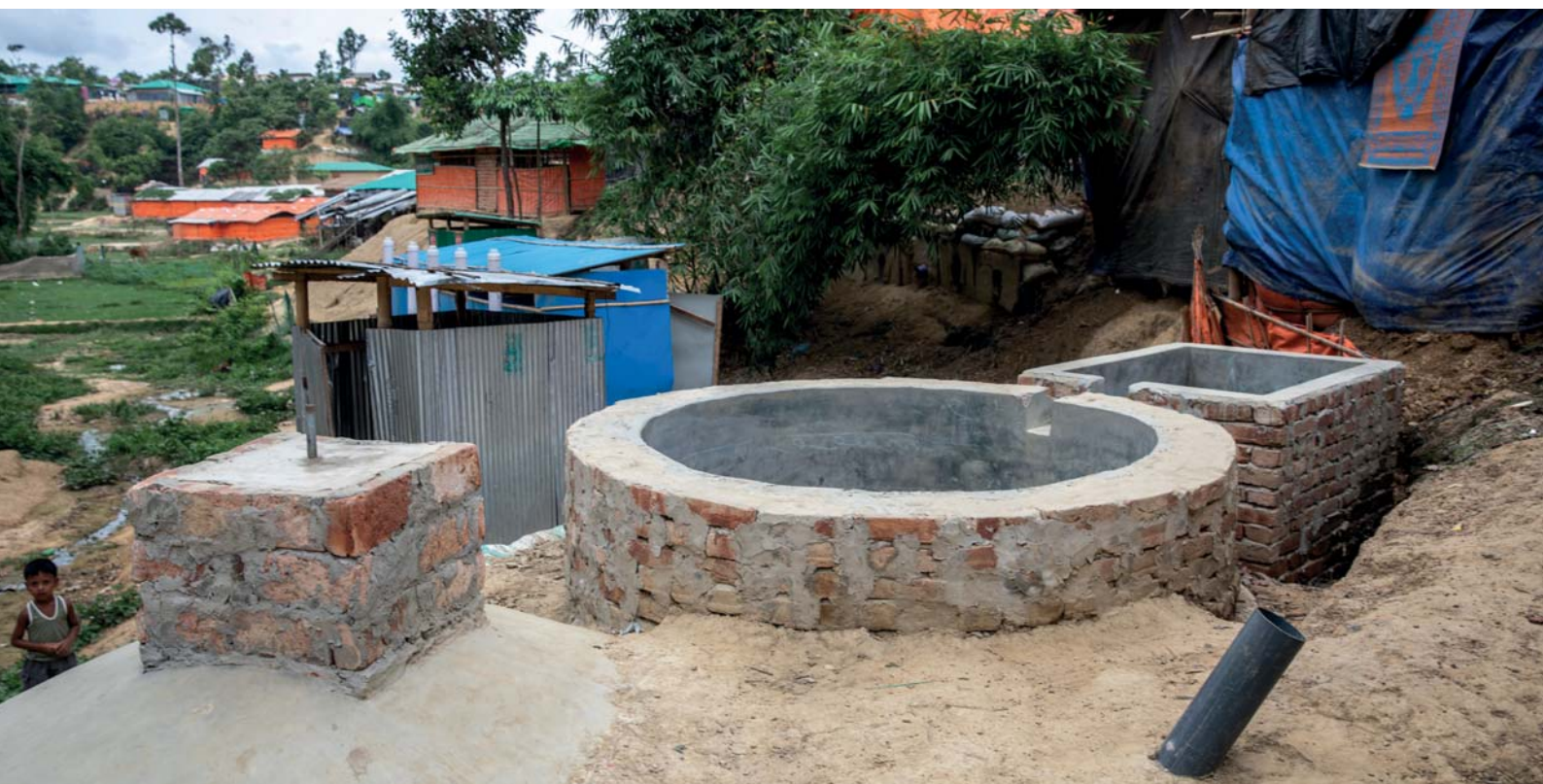
The biogas plants consist of a biogas reactor, a hydraulic chamber and a slurry pit.
