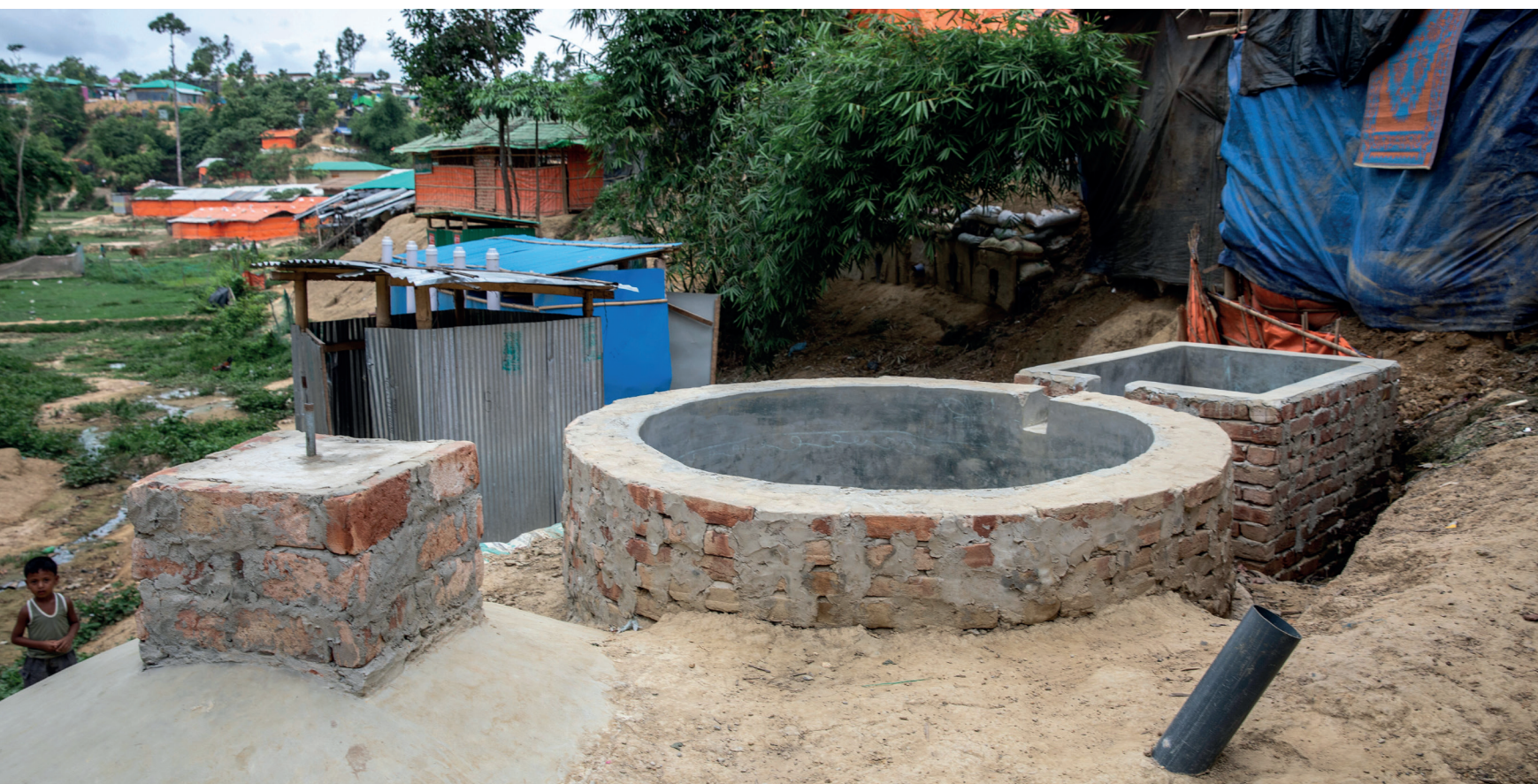
The biogas plants consist of a biogas reactor, a hydraulic chamber and a slurry pit.
