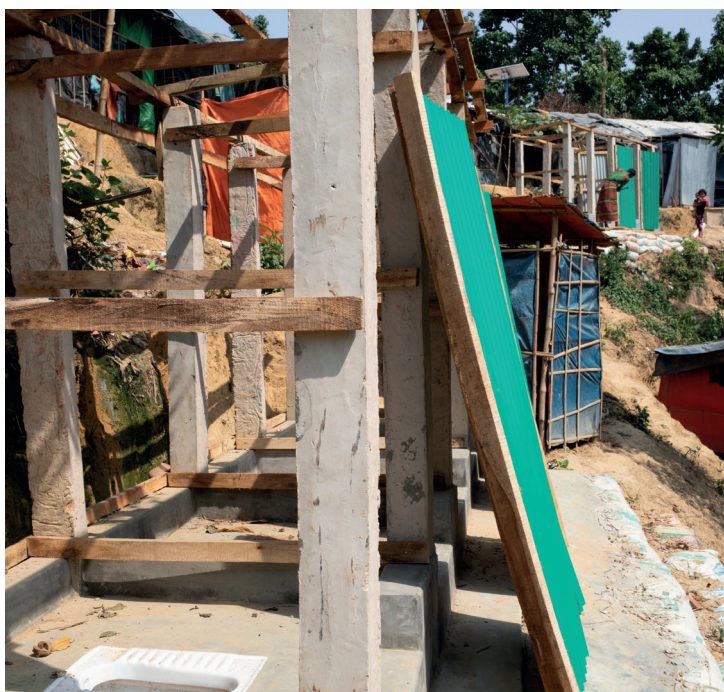
Forty latrine blocks of five to eight cabins, each connected to twelve sets of biogas plants with a kitchen, were installed.
