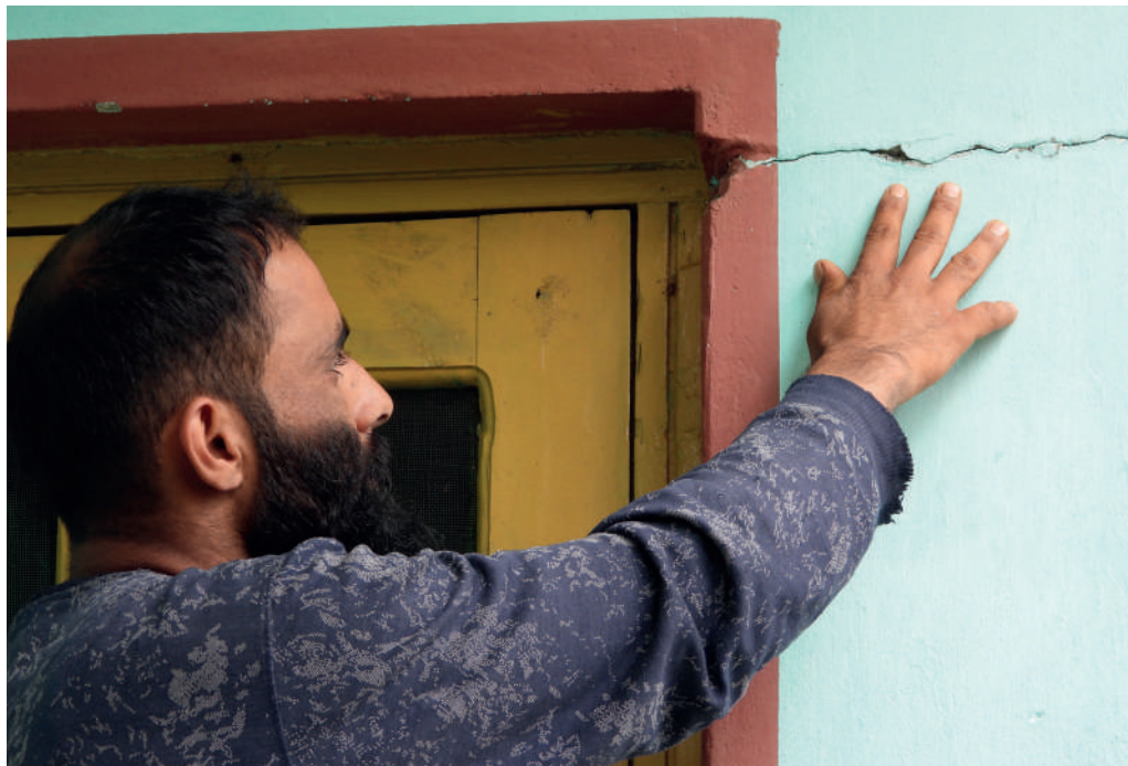
A villager in Kashmir Himalayas showing the crack in the outer wall of his house.
