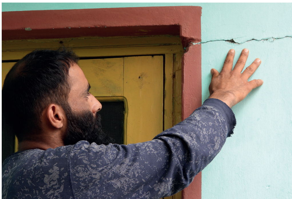
A villager in Kashmir Himalayas showing the crack in the outer wall of his house.
